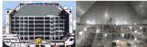
Figure 1: A Typical membrane-type LNG cargo hold system scaffolding
